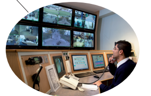
CCTV / digital recorder integration
